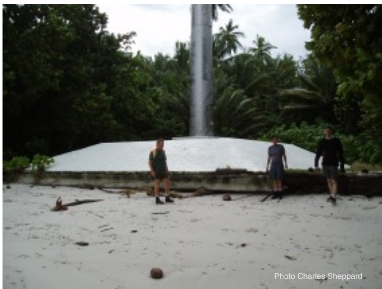
Eastern Diego Garcia, lagoon shore, where a large navigation marker now abuts the beach with undercutting of its foundation.
